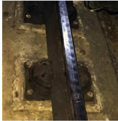
Fig. 2. Picture of corrugation on-site
