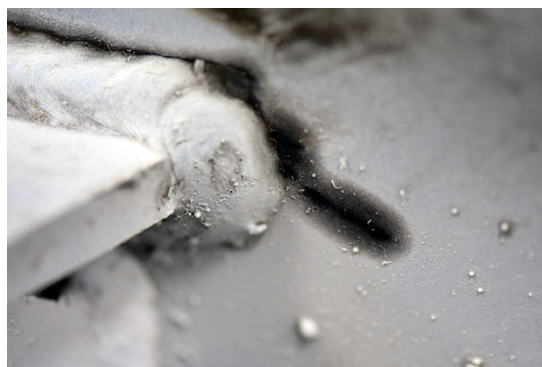
Fig. 9. Hair cracks in a component made of high-strength steel (S700MC) using dye-penetrant technique after 2 \times 10^6 cycles.
