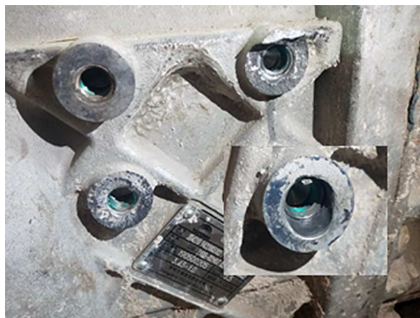
Fig. 1. Rupture position of the support hole
