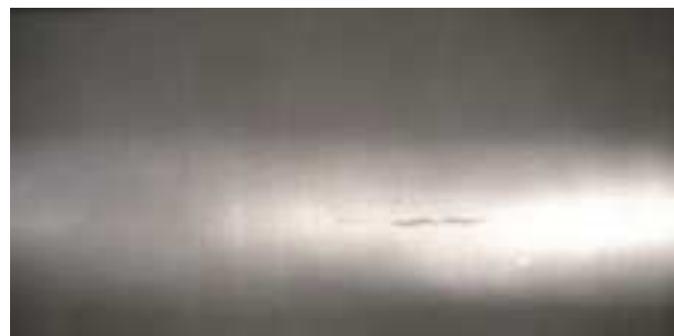
Fig. 1. The steel plate with a surface crack
